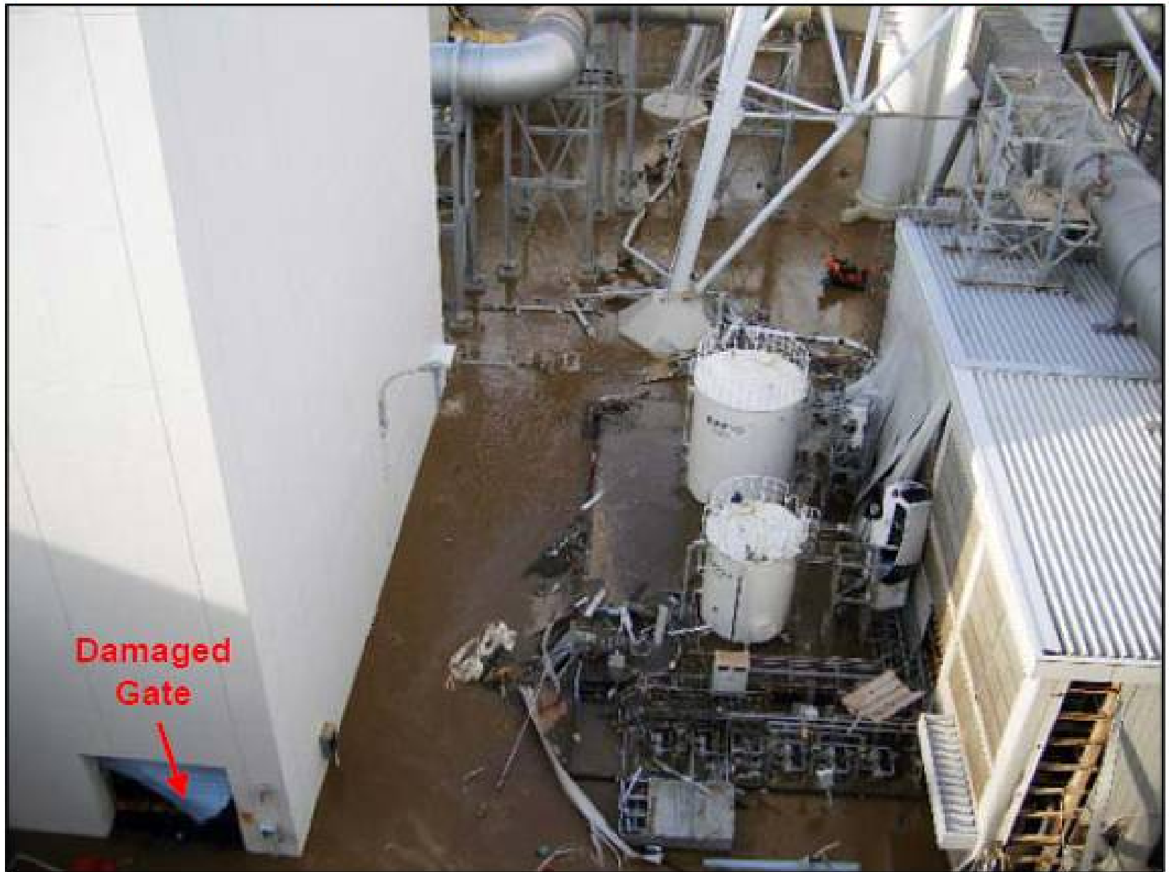
4 to 5 m inundation height across reactor and turbine buildings.
